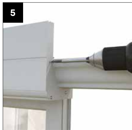
5 CORNICE & FLY THROUGH GUTTER DETAIL - Used when the gutter extends beyond the Cornice. Take the end plate and cut to the shape of the gutter that projects beyond the Cornice.
