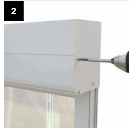
2 GUTTER STOP END DETAIL - Used with lean-to roofs, gable roofs or when the gutter returns along the host wall. Secure the end plate into position using the fixings provided (CRN008).
