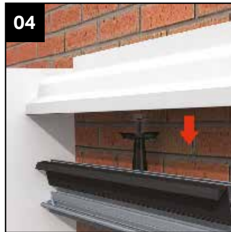
04 Now clip on the wallplate PVCu top cap, mark out for the flashing and grind out.
