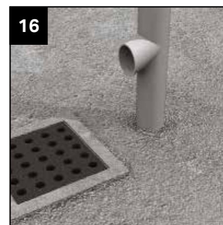
16 Ensure pitch is correct and structure is square. Fill holes around posts with appropriate concrete mix.
