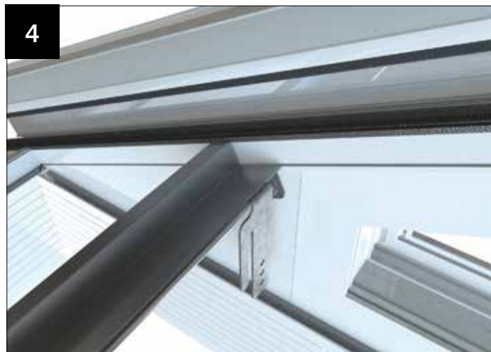
4 Offer into position the cloaking panel support trim - the nose of the closure trim must be notched back as shown (at the gable side only).
