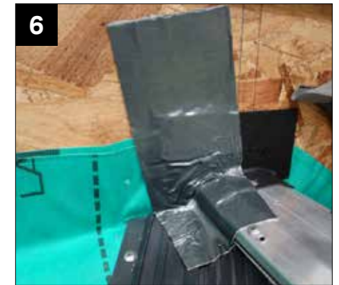
6 Image shows examples where 1 Butyl patch is applied - Glazing on duo-pitch segment (main image) and glazing on lean-to segment (inset image)
