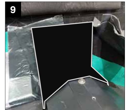
9 Fit the supplied host wall flashing cap using a low modulus silicone.
