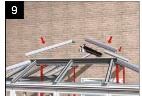
Using the roof location plan, build the upper roof as per section 4 of this guide.
