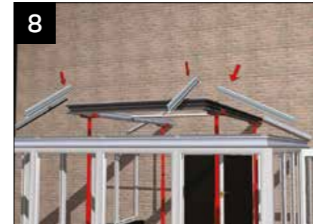
Now the Pagoda eaves beam is assembled into a one piece structure, temporarily support it. Attach the glazing bars according to the component location plan. Tighten the bars, at the pagoda beam end first and then at the main eaves beam second. At the corners, seal using a sealant appropriate to the glazing material (shown above).
