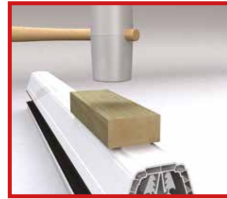
44 Knock the glazing bar top cappings on with a Deadblow hammer. Greater care is needed in cold weather. Keep all trims wrapped until they are needed. Once again each capping is numbered according to its position in the roof.
