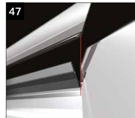
48 Ensure the jack rafter top capping is lined up correctly (as above) before knocking the top cappings into position. It is not possible to 'tap up' the jack rafter top caps into final position when fitted with anchor clips.
