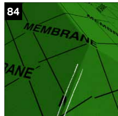
With the spine removed. Continue to follow fitting of the tile starter strips.
