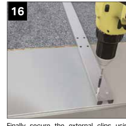
Finally secure the external clips using WPCS020 4.8mm x 38mm self drilling screws provided. NOTE: do not stand on the panels to secure the external clips. Tip: on greater projections secure the clip to the beam (as step 16). Then fit the first row of OSB boarding, this will allow easier access to secure the panel clips further up the roof.
