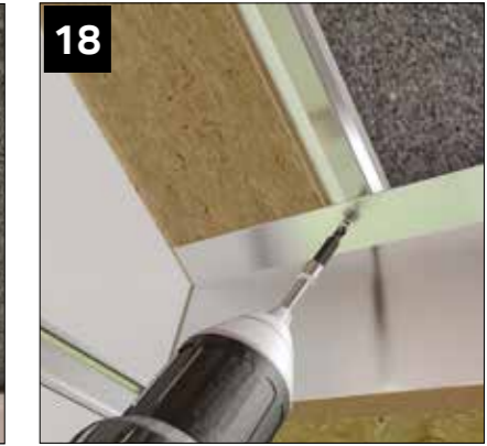
Secure the gable end panel (s) only by screwing up through the box beam shelf and the upper half ridge shelf using 1 x NRTS050 screws provided.
