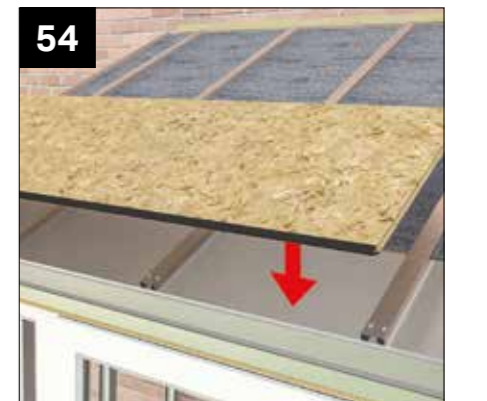
Following location plan, locate first row of OSB panels around the roof using tile starter support section to position. Ensure OSB sheets are the right way up, orientation.
