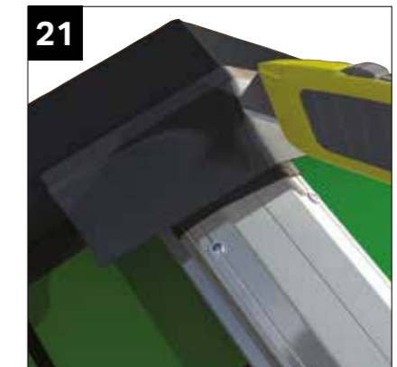
21 Fit second 200mm Butyl tape sealing the dry verge to the gable flashing. Cut the tape to allow it to be folded as shown in the following two images
