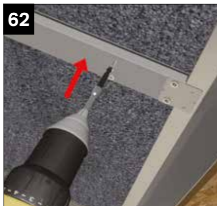
62 Secure into the panel (at box beam end) as previous image. Again, note method of alternate tightening sequence 63-65.
