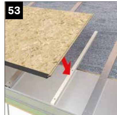
Where required support OSB board at butt joints using timber battens supplied. Battens are 65 x 19 x 700mm long (NRPB010). Only required over box beam using the screws provide WPCS 020 (2 x per batten).
