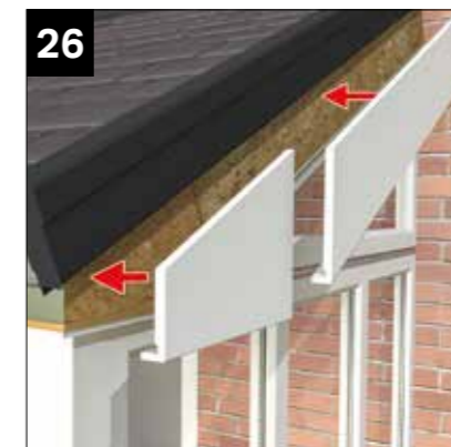
26 Fit the pre-cut fascia and eaves trims. See page 50, images 44 to 47 for more detail.
