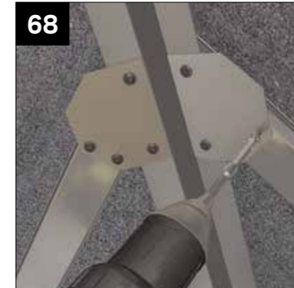
68 Where jack rafter abuts hip bar fix the jack rafter connection plates using 4 x CHAA 006 screws provided. NOTE: fit one screw through half clip that meets hip bar.
