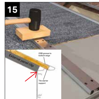
When aligned (ensure external panel clip butts upto aluminium gutter channel, see red arrow) use a robust mallet to knock down the external panel locking clips (use a short length of timber to protect the clip from indentations).
