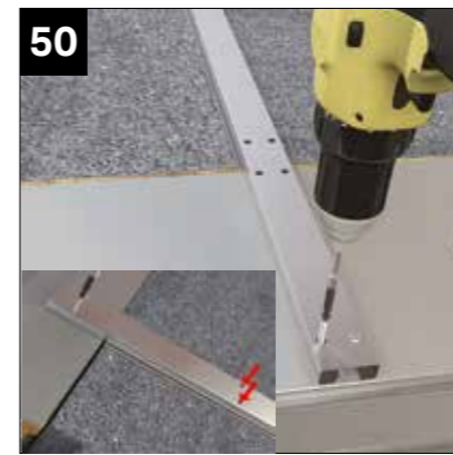
Finally secure the external clips using WPCS020 4.8mm x 38mm self drilling screws provided. (2 into ridge section, 4 into panels and 4 into box beam on full length clips) or through pre-drilled holes on short clips or half clips.
